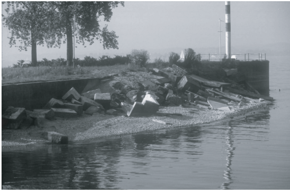
Fig. 4. Damaged shore fortifications on the eastern shore of Lake Constance near Bregenz.
