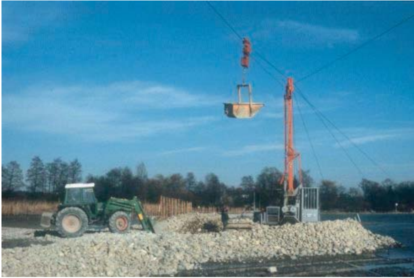
Fig. 5. Lakeshore rehabilitation works during low water period in February. Here, an eroded beach is filled up with a basement of boulders to give a break wave construction.
